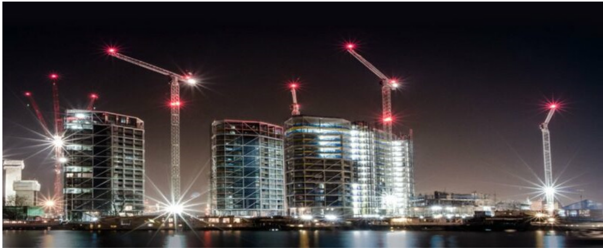
Figure 5 Typical Examples of Crane Aviation Warning Lighting
